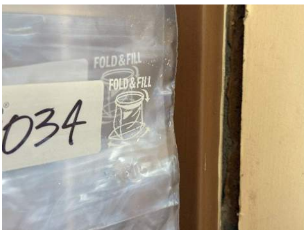
Samples 033 / 034 Door Caulk Site/Office Building, 2 nd Floor Interior @ North No asbestos detected
