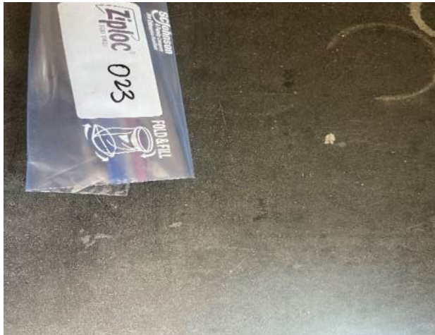
Samples 023 / 024 Black Countertop Site/Office Building, 2 nd Floor Lab 10% Chrysotile
