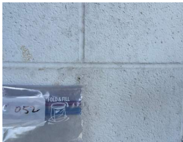
Samples 052 / 053 CMU & Paint Texture Site/Office Building, Exterior No asbestos detected
