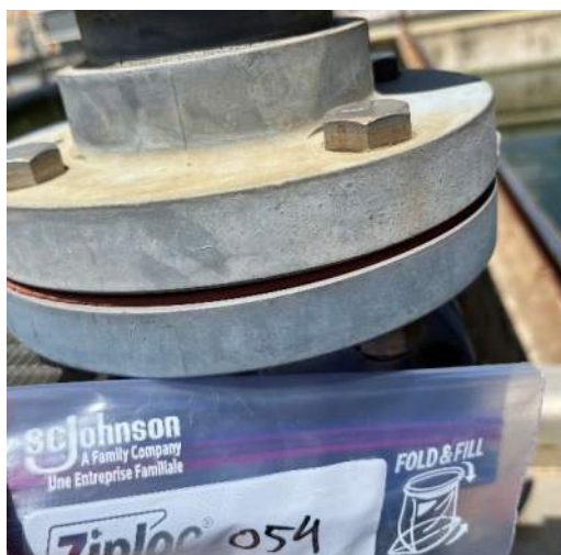
Samples 054 / 055 Red Rubber Gasket Chlorine Contact Chamber & Valves No asbestos detected
